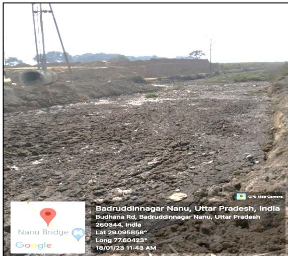
Figure 71 Sardhana drain covered with layer of cattle dung
