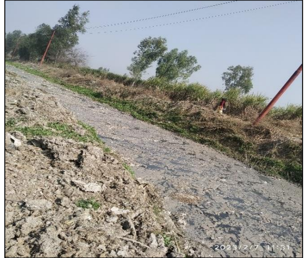
Figure 47 Sludge deposition in Jat Mujheda drain
