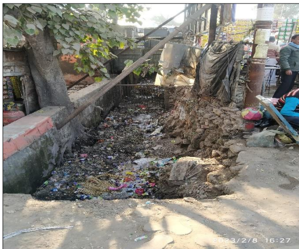
Figure 34 Shamli Road drain at origin (dumping of solid waste in drain)
