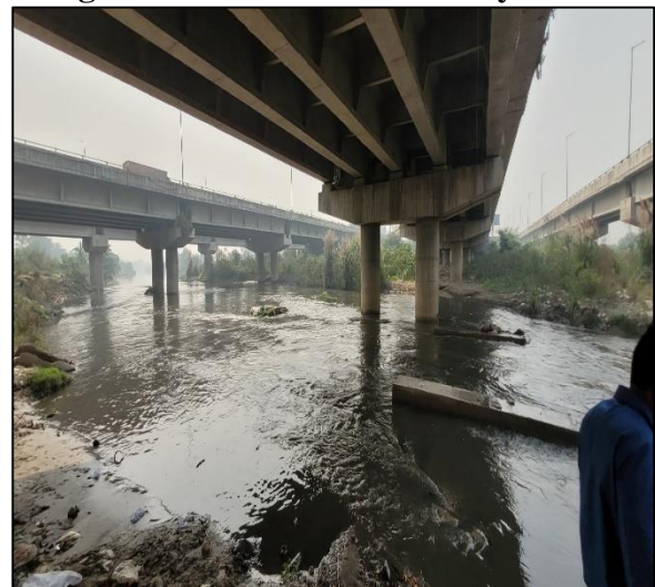
Figure 97 Hindon A/c Dasna drain
